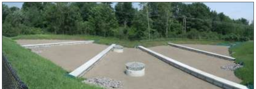
Completed underdrained soil filter. Stormwater is collected from the Mall Plaza site and distributed through a junction box to the separate cells. Overflow outlets (concrete structures with beehive covers) are designed to control runoff from storms greater than one inch.
