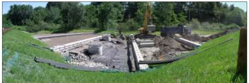
Underdrained soil filter under construction. Each cell is comprised of geotextile filter fabric, a 12 inch layer of drainage stone and underdrain piping, and an 18 inch layer of soil media that provide the effective absorption of pollutants and fine sediment removal.
