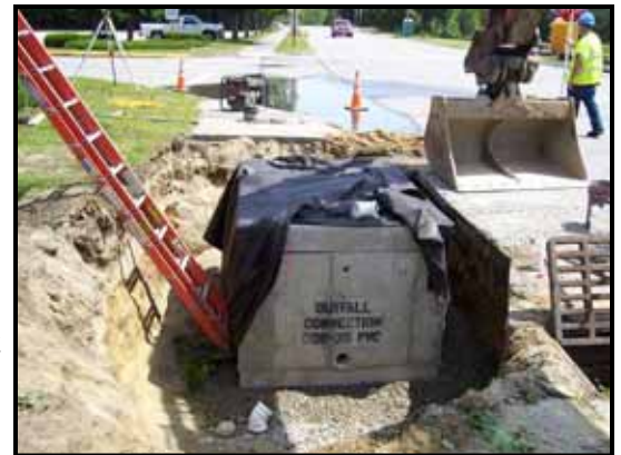
Installation of a Filterra tree box at an existing catch basin on Philbrook Avenue in South Portland.
