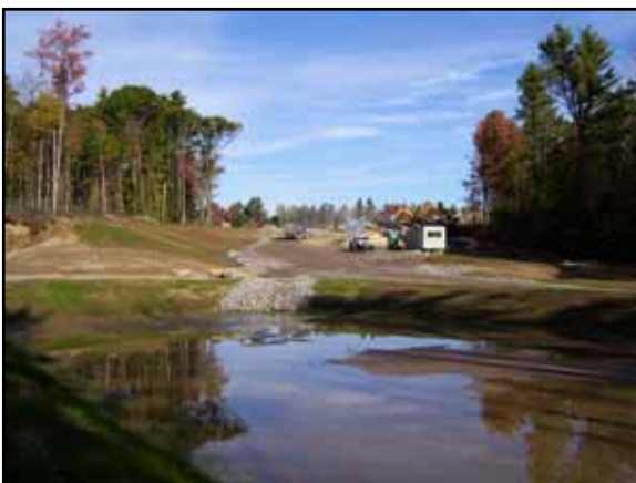
Contractors certified through the VCCP implement best management practices such as encouraging revegetation and filtering of site runoff.
