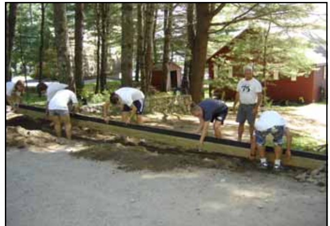
The Little Sebago Lake YCC installs a rubber razor blade to divert driveway runoff.
