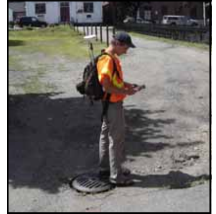
An intern uses GPS technology to document the location of a storm drain.
