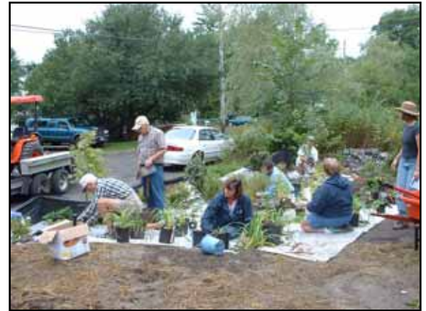
Volunteers install a rain garden in the Highland Lake Watershed in Windham.
